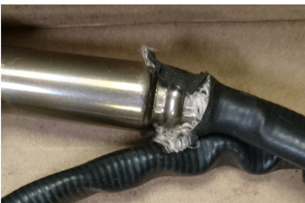
Figure 14. Evidence of damaged wiring.
